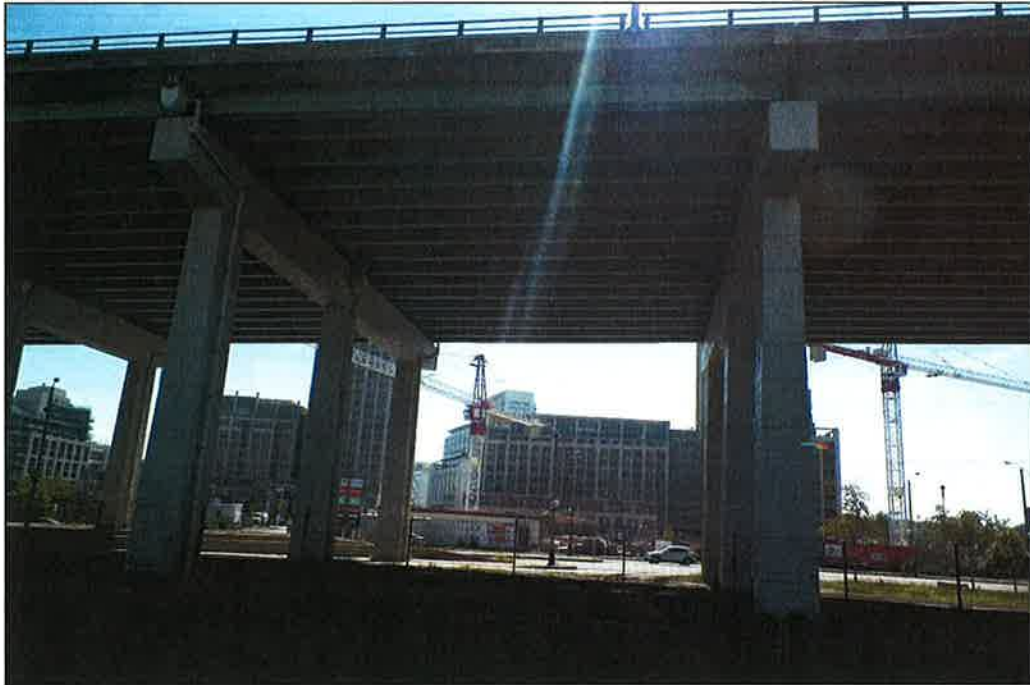
Photo P17 – Elevation (Bent 91-92) (fair condition – stained and unstained cracking, delaminations, isolated spalls, patches, wet areas and light scaling)
