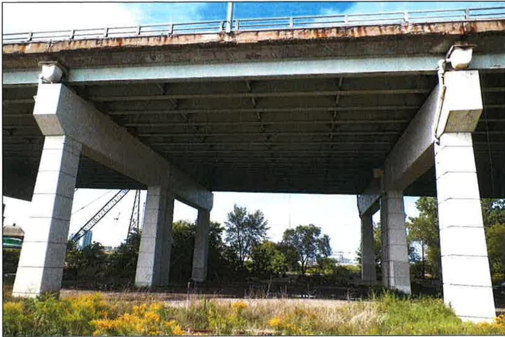
Photo P41 – Elevation (Bent 301-302) (fair-to-poor condition – stained and unstained cracking, delaminations, spalls, patches, wet areas and light scaling)
