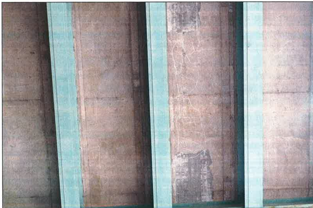
Photo P22 – Typical Condition of Soffit (Bent 91-92) (fair condition – stained and unstained cracking, delaminations, isolated spalls, patches, wet areas and light scaling)
