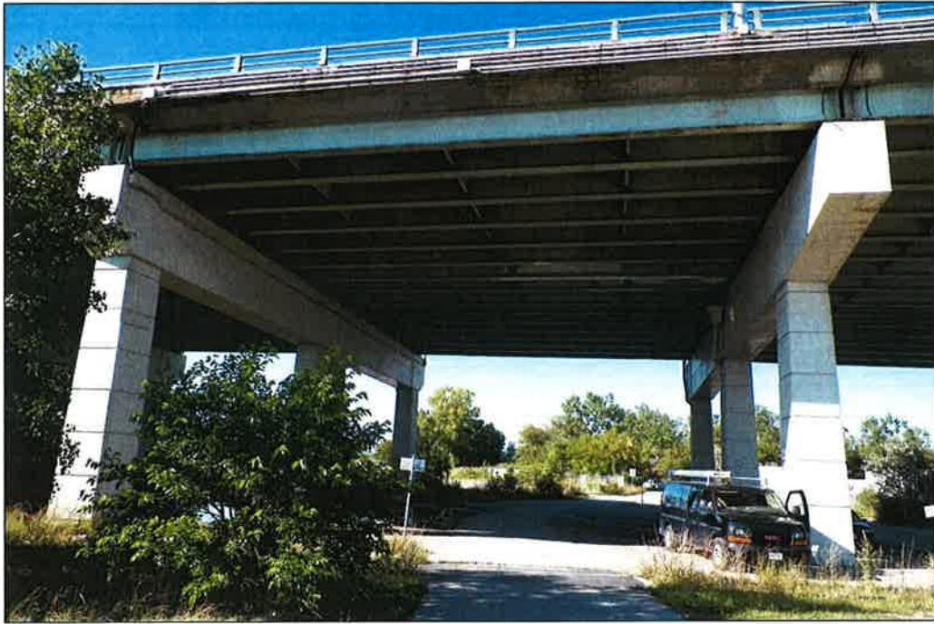
Photo P49 – Elevation (Bent 306-307) (fair condition – stained and unstained cracking, delaminations, spalls, patches, wet areas and light scaling)
