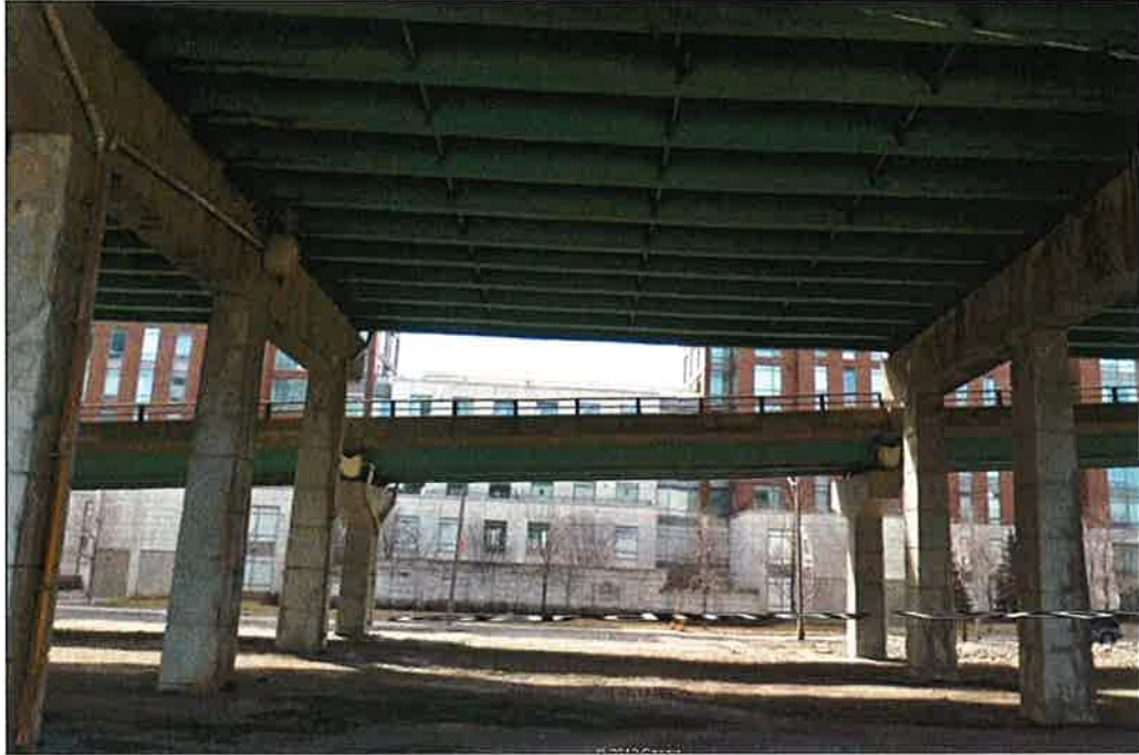
Photo P25 – Elevation (Bent 120-121) (fair condition – stained and unstained cracking, isolated delaminations and spalls, patches and light scaling)
