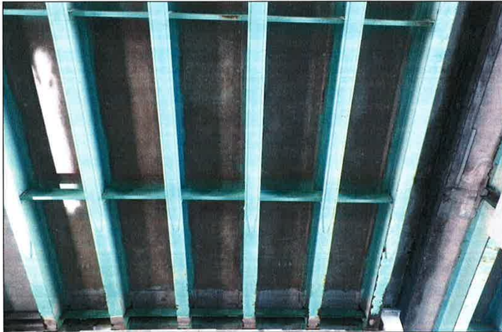
Photo P30 – Typical Condition of Soffit (Bent 120-121) (fair condition – stained and unstained cracking, isolated delaminations and spalls, patches and light scaling)
