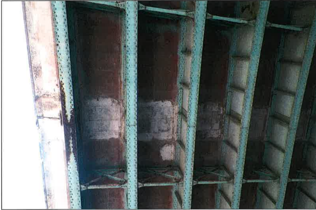
Photo P37 – Typical Condition of Soffit (Bent 131-132) (fair condition – stained and unstained cracking, isolated delaminations and spalls, patches and light scaling)
