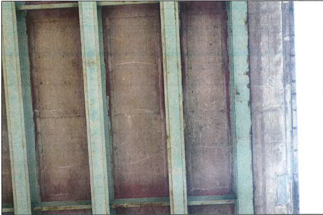
Photo P13 – Typical Condition of Soffit (Bent 85-86) (fair condition – stained and unstained cracking, delaminations and patches)
