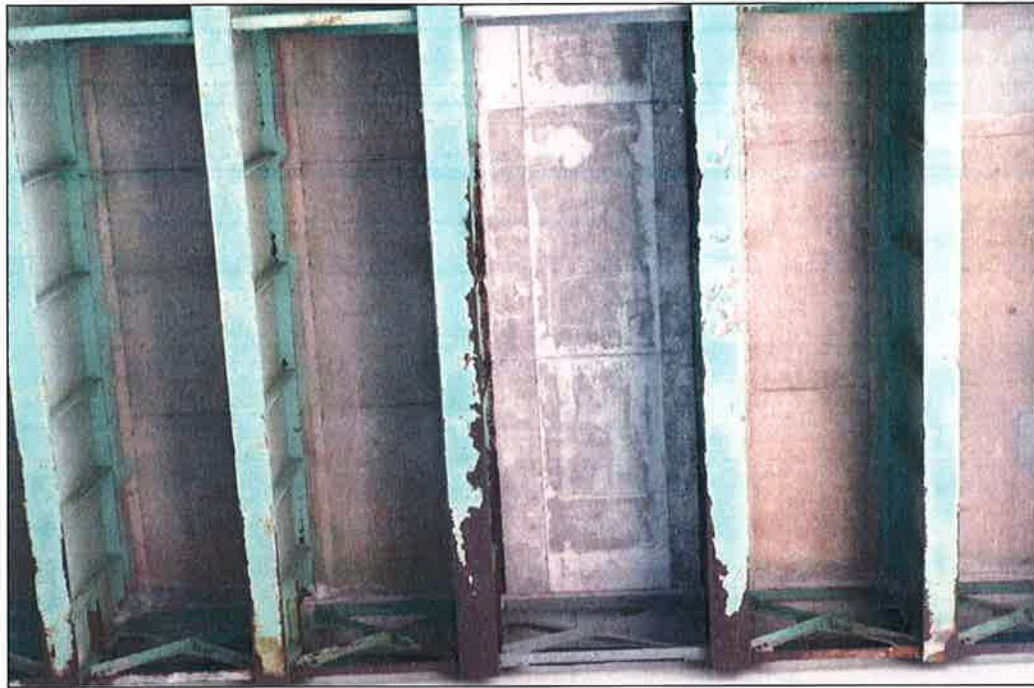
Photo P5 – Typical Condition of Soffit (Bent 53-55) (fair condition – stained and unstained cracking, delaminations, isolated spalls, patches, wet areas and light scaling)
