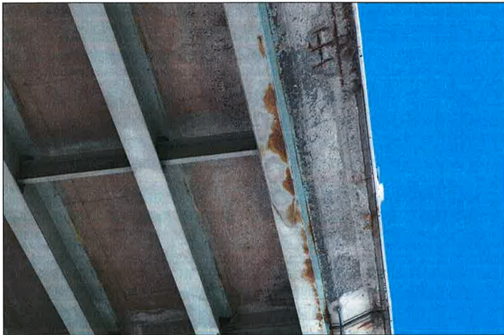
Photo P52 – Typical Condition of Soffit (Bent 306-307) (fair condition – stained and unstained cracking, delaminations, spalls, patches, wet areas and light scaling)
