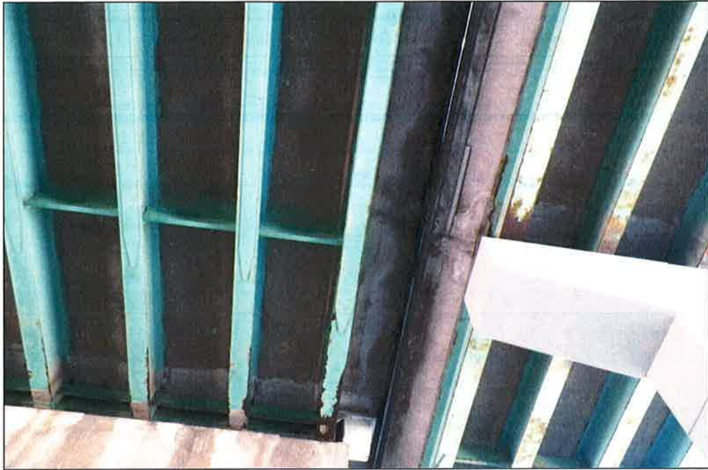
Photo P31 – Typical Condition of Soffit (Bent 120-121) (fair condition – stained and unstained cracking, isolated delaminations and spalls, patches and light scaling)
