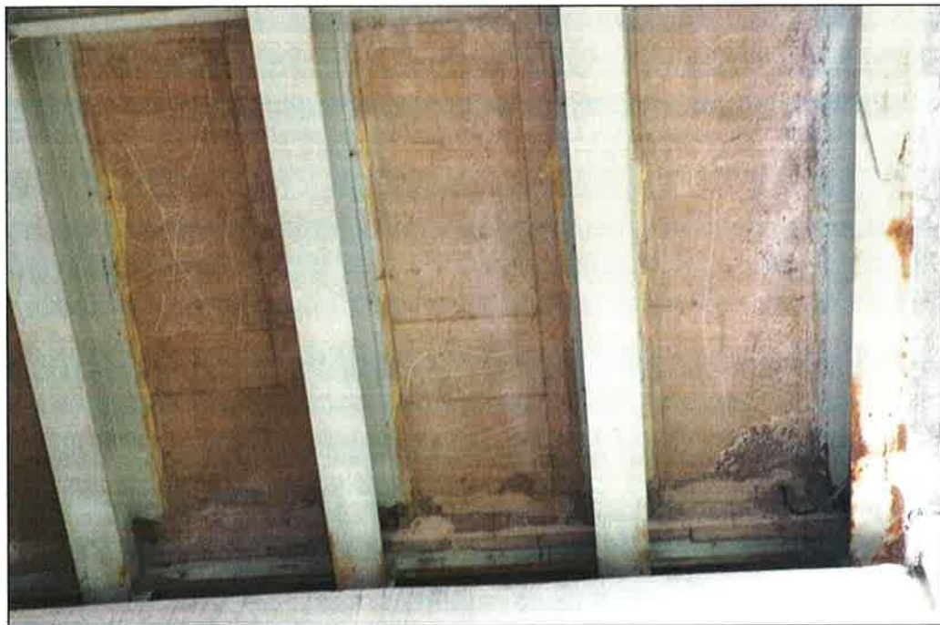
Photo P46 – Typical Condition of Soffit (Bent 301-302) (fair-to-poor condition – stained and unstained cracking, delaminations, spalls, patches, wet areas and light scaling)
