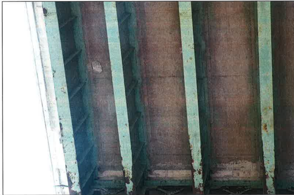
Photo P4 – Typical Condition of Soffit (Bent 53-55) (fair condition – stained and unstained cracking, delaminations, isolated spalls, patches, wet areas and light scaling)
