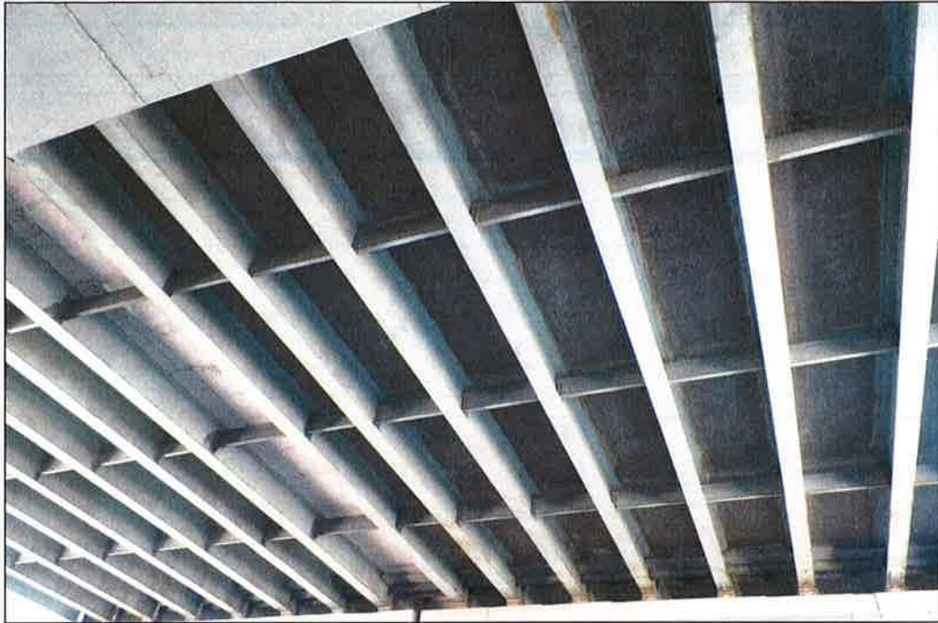
Photo P51 – Typical Condition of Soffit (Bent 306-307) (fair condition – stained and unstained cracking, delaminations, spalls, patches, wet areas and light scaling)
