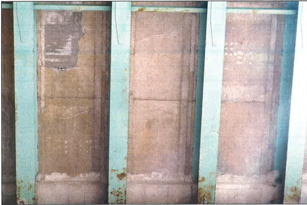
Photo P21 – Typical Condition of Soffit (Bent 91-92) (fair condition – stained and unstained cracking, delaminations, isolated spalls, patches, wet areas and light scaling)
