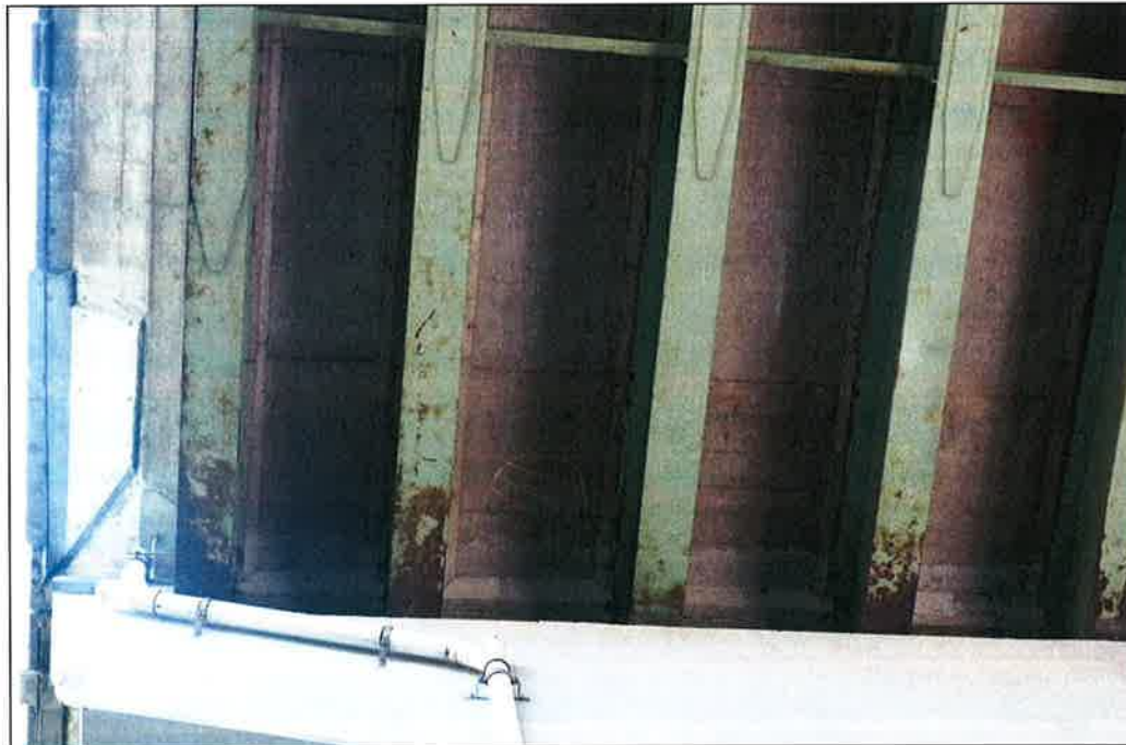
Photo P12 – Typical Condition of Soffit (Bent 85-86) (fair condition – stained and unstained cracking, delaminations and patches)
