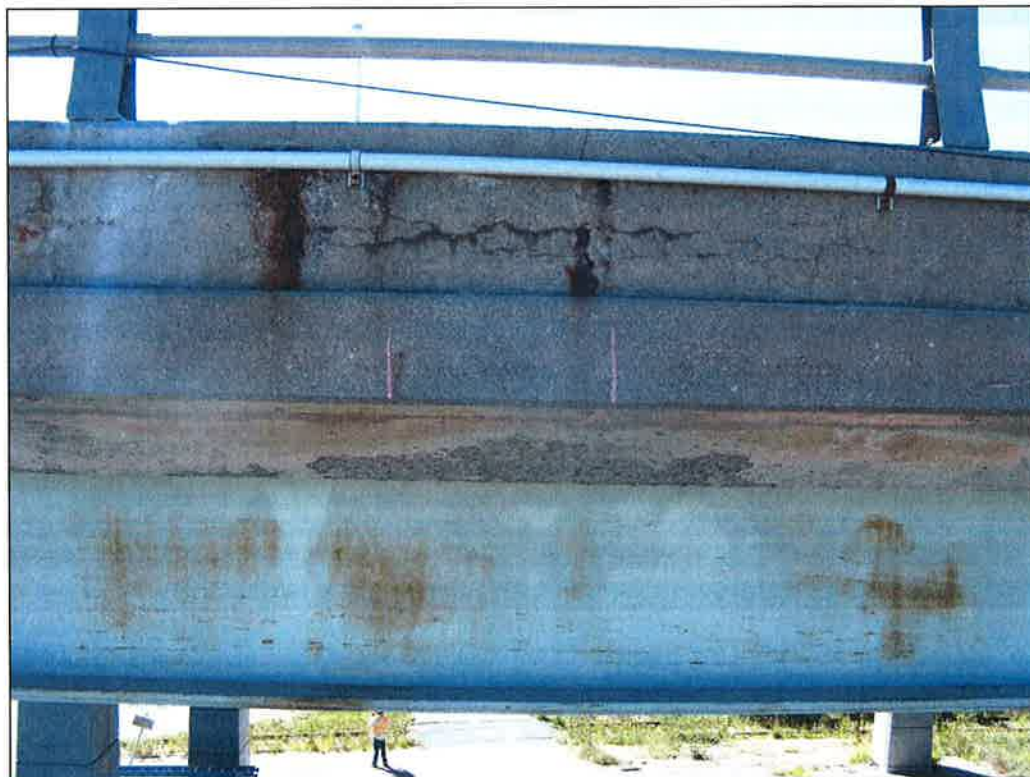
Photo P56 – Typical Condition of Fascia (Bent 306-307) (poor condition – cracking, spalls and localized patches)
