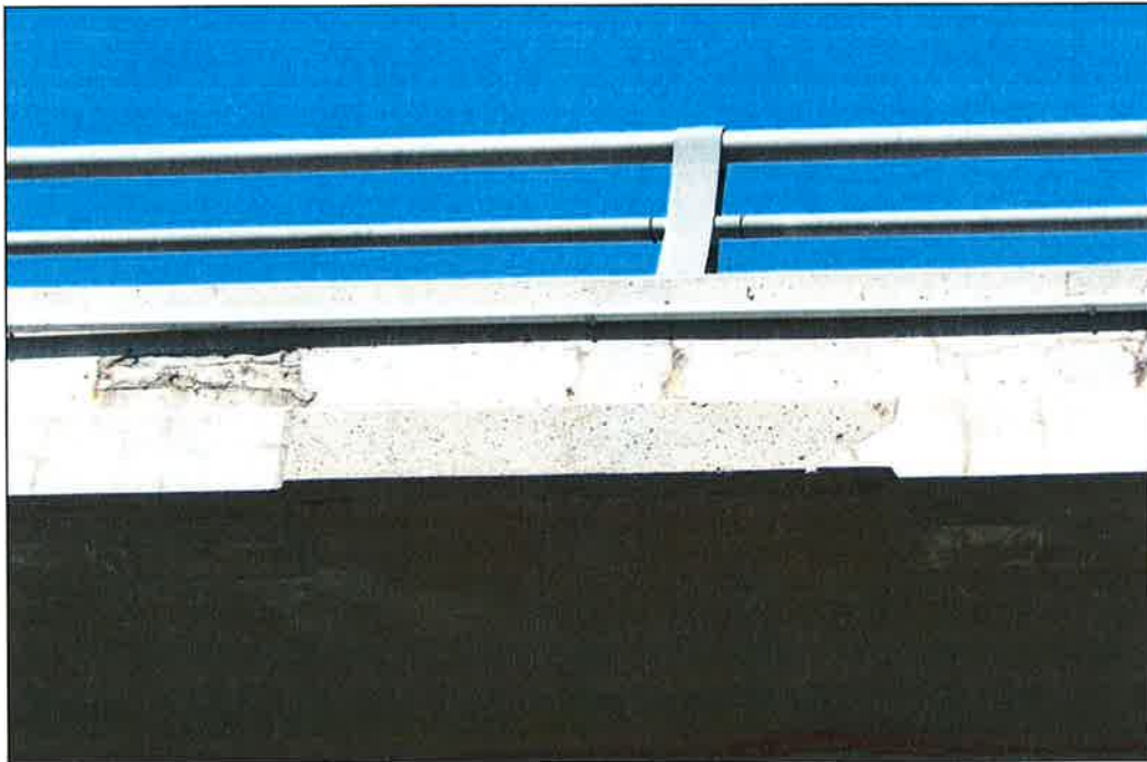
Photo P16 – Typical Condition of Fascia (Bent 85-86) (fair condition –cracking, isolated delaminations and patches)
