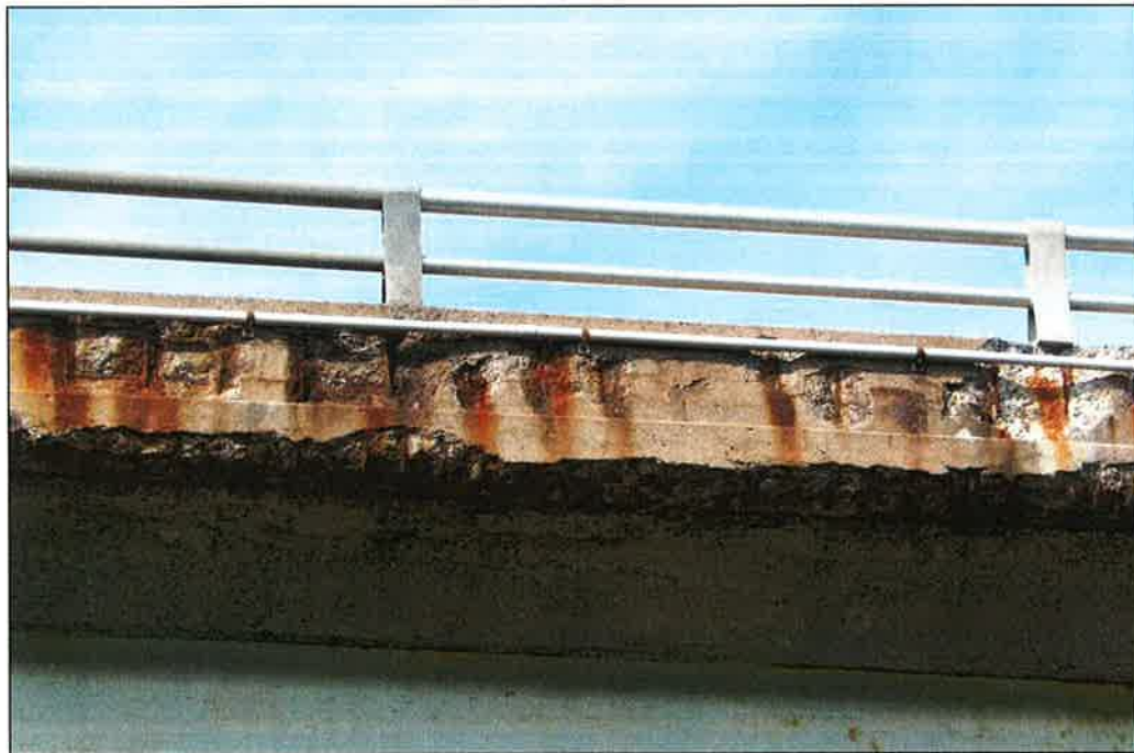
Photo P48 – Typical Condition of Fascia (Bent 301-302) (poor condition –cracking, delaminations and spalls)
