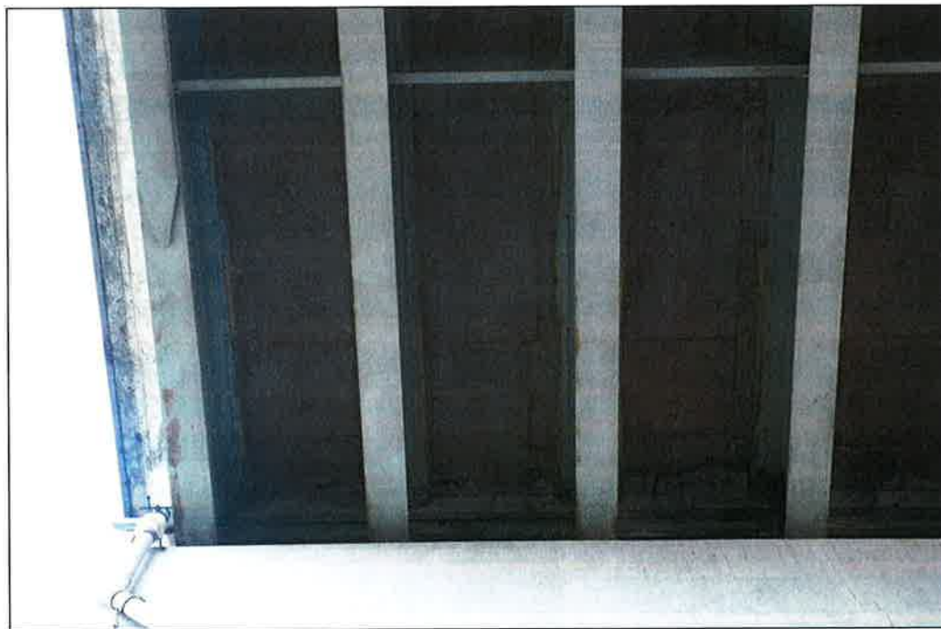
Photo P44 – Typical Condition of Soffit (Bent 301-302) (fair-to-poor condition – stained and unstained cracking, delaminations, spalls, patches, wet areas and light scaling)
