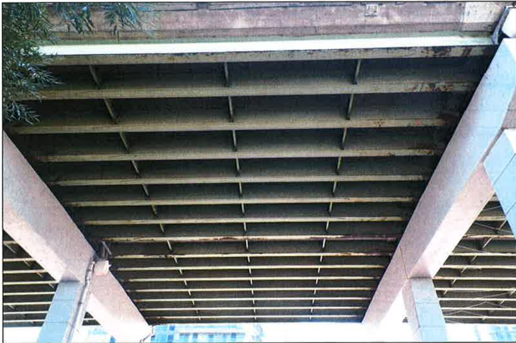
Photo P11 – Typical Condition of Soffit (Bent 85-86) (fair condition – stained and unstained cracking, delaminations and patches)
