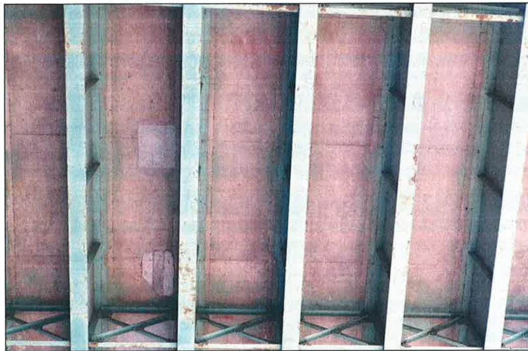
Photo P6 – Typical Condition of Soffit (Bent 53-55) (fair condition – stained and unstained cracking, delaminations, isolated spalls, patches, wet areas and light scaling)
