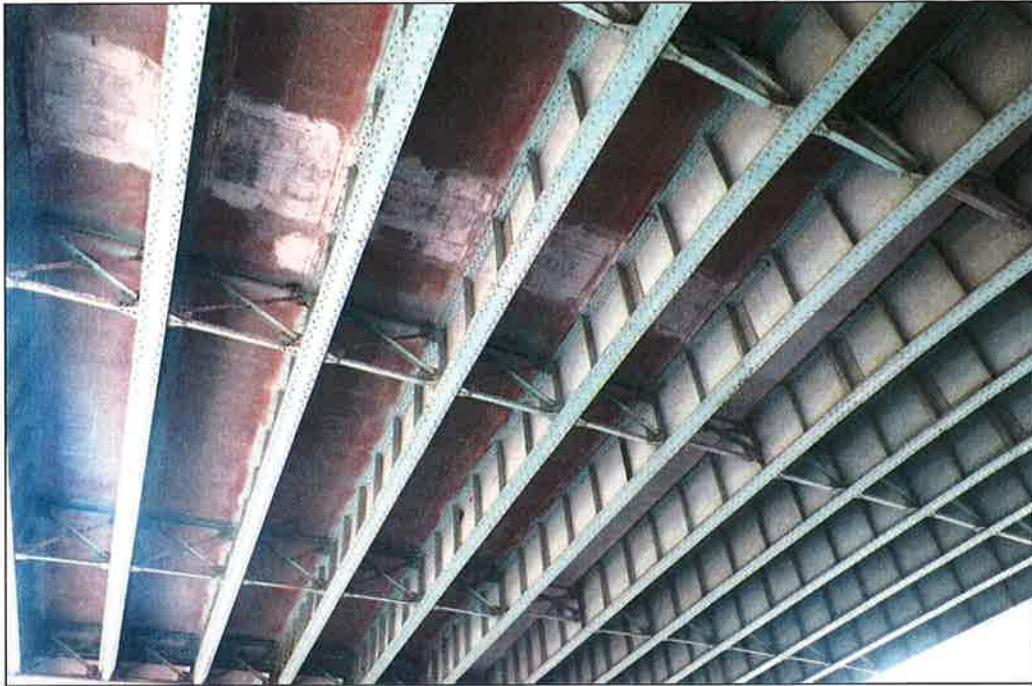
Photo P35 – Typical Condition of Soffit (Bent 131-132) (fair condition – stained and unstained cracking, isolated delaminations and spalls, patches and light scaling)
