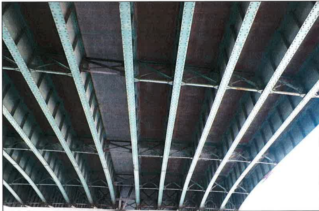
Photo P36 – Typical Condition of Soffit (Bent 131-132) (fair condition – stained and unstained cracking, isolated delaminations and spalls, patches and light scaling)
