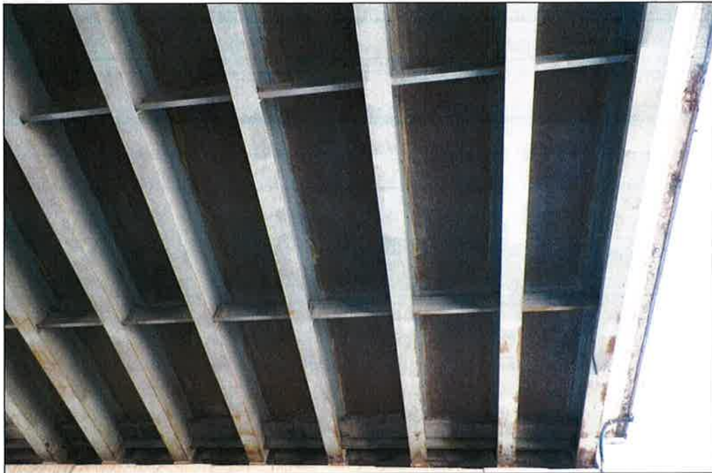
Photo P55 – Typical Condition of Soffit (Bent 306-307) (fair condition – stained and unstained cracking, delaminations, spalls, patches, wet areas and light scaling)
