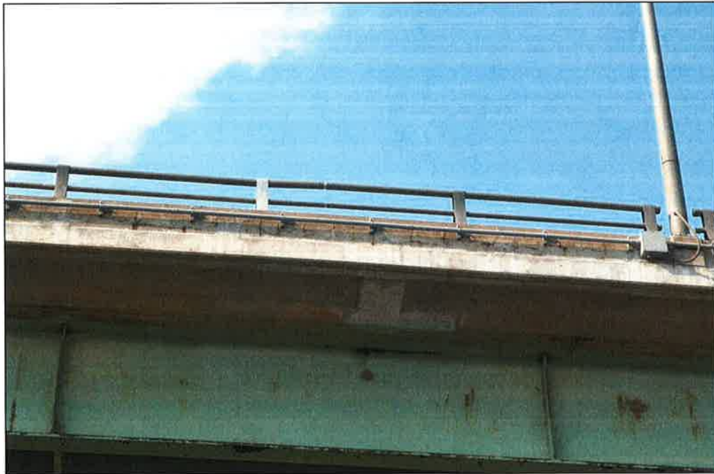
Photo P8 – Typical Condition of Fascia (Bent 53-55) (fair condition –cracking and patches)
