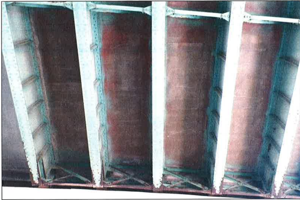
Photo P39 – Typical Condition of Soffit (Bent 131-132) (fair condition – stained and unstained cracking, isolated delaminations and spalls, patches and light scaling)
