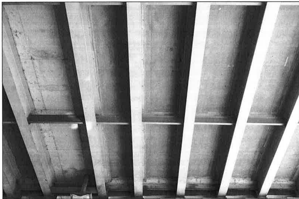
Photo P54 – Typical Condition of Soffit (Bent 306-307) (fair condition – stained and unstained cracking, delaminations, spalls, patches, wet areas and light scaling)
