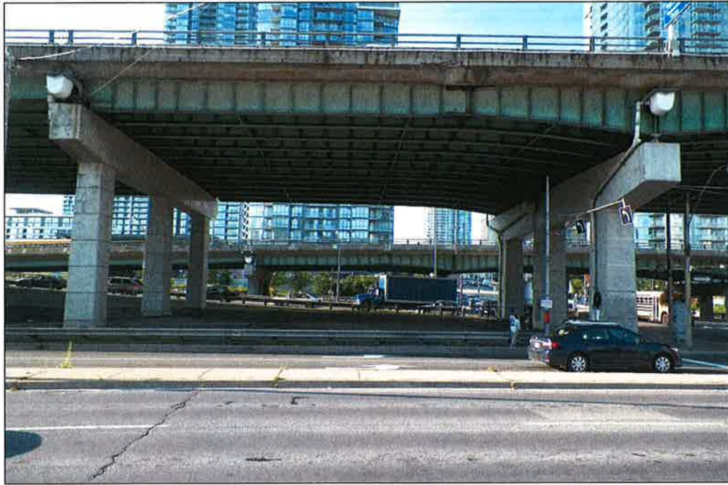
Photo P33 – Elevation (Bent 131-132) (fair condition – stained and unstained cracking, isolated delaminations and spalls, patches and light scaling)
