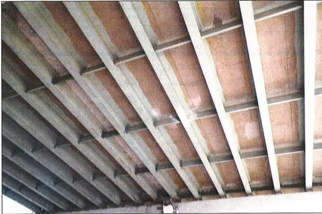
Photo P43 – Typical Condition of Soffit (Bent 301-302) (fair-to-poor condition – stained and unstained cracking, delaminations, spalls, patches, wet areas and light scaling)
