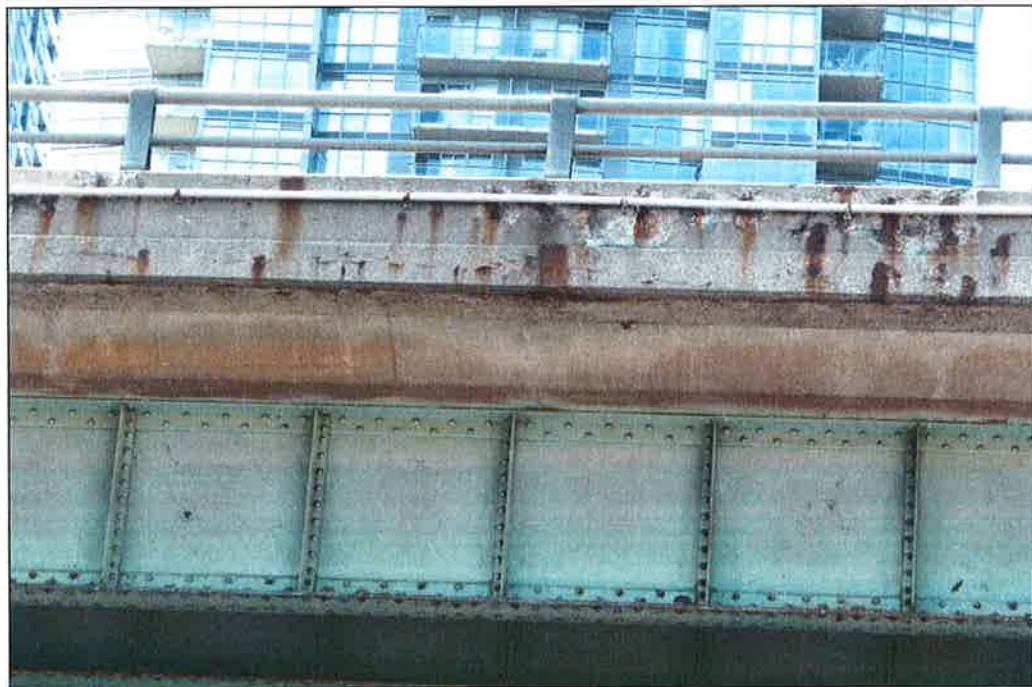
Photo P40 – Typical Condition of Fascia (Bent 131-132) (poor condition – cracking, delaminations, spalls and isolated patches)
