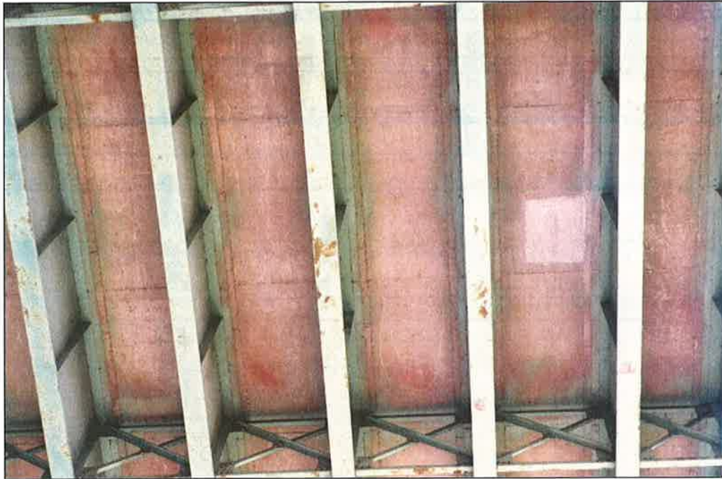
Photo P7 – Typical Condition of Soffit (Bent 53-55) (fair condition – stained and unstained cracking, delaminations, isolated spalls, patches, wet areas and light scaling)
