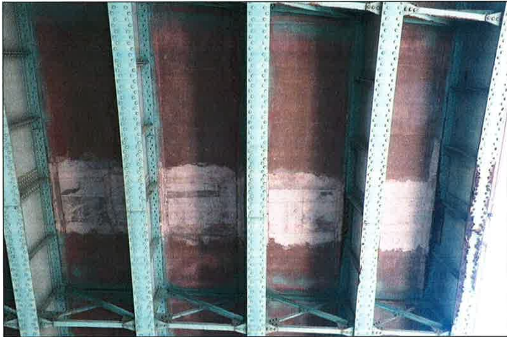
Photo P38 – Typical Condition of Soffit (Bent 131-132) (fair condition – stained and unstained cracking, isolated delaminations and spalls, patches and light scaling)
