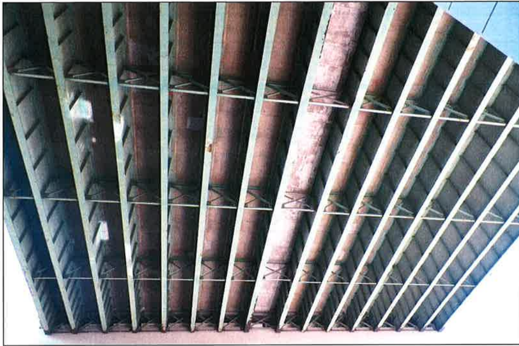
Photo P3 – Typical Condition of Soffit (Bent 53-55) (fair condition – stained and unstained cracking, delaminations, isolated spalls, patches, wet areas and light scaling)
