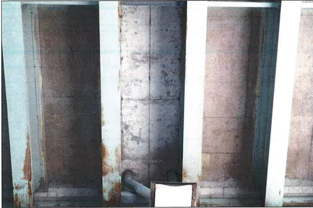
Photo P45 – Typical Condition of Soffit (Bent 301-302) (fair-to-poor condition – stained and unstained cracking, delaminations, spalls, patches, wet areas and light scaling)
