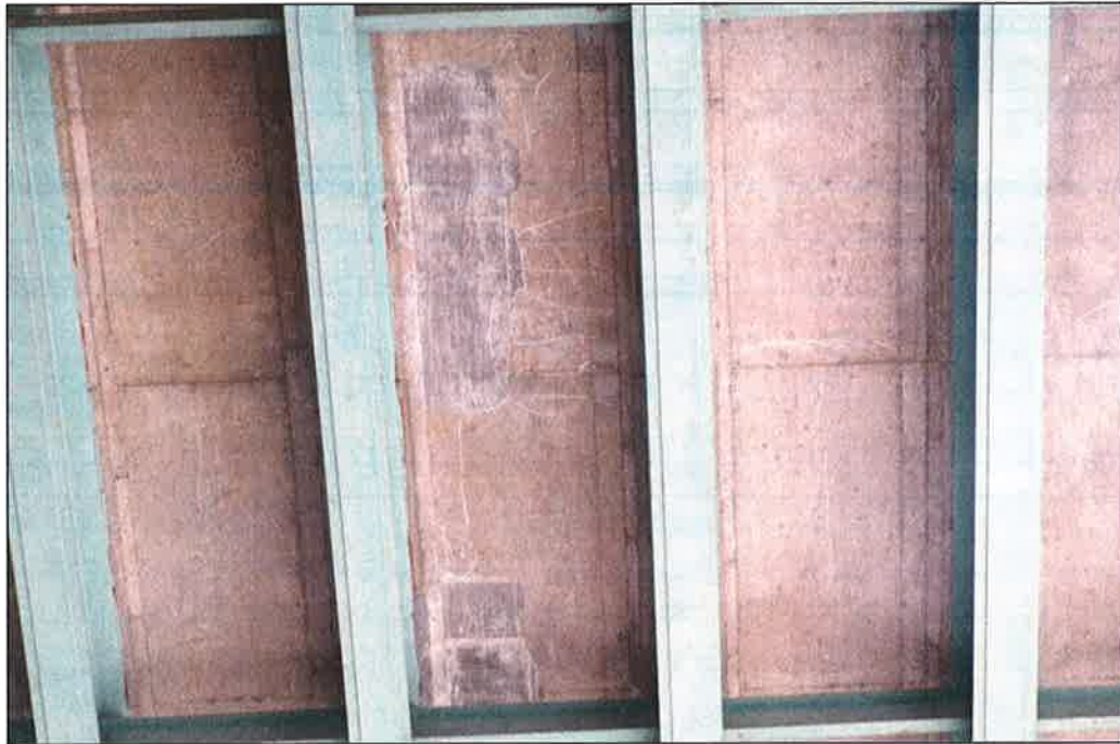
Photo P23 – Typical Condition of Soffit (Bent 91-92) (fair condition – stained and unstained cracking, delaminations, isolated spalls, patches, wet areas and light scaling)
