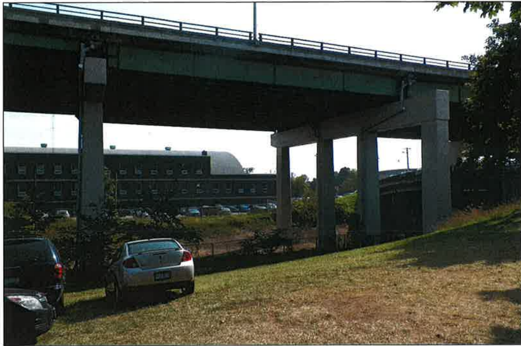
Photo P1 – Elevation (Bent 53-55) (fair condition – stained and unstained cracking, delaminations, isolated spalls, patches, wet areas and light scaling)
