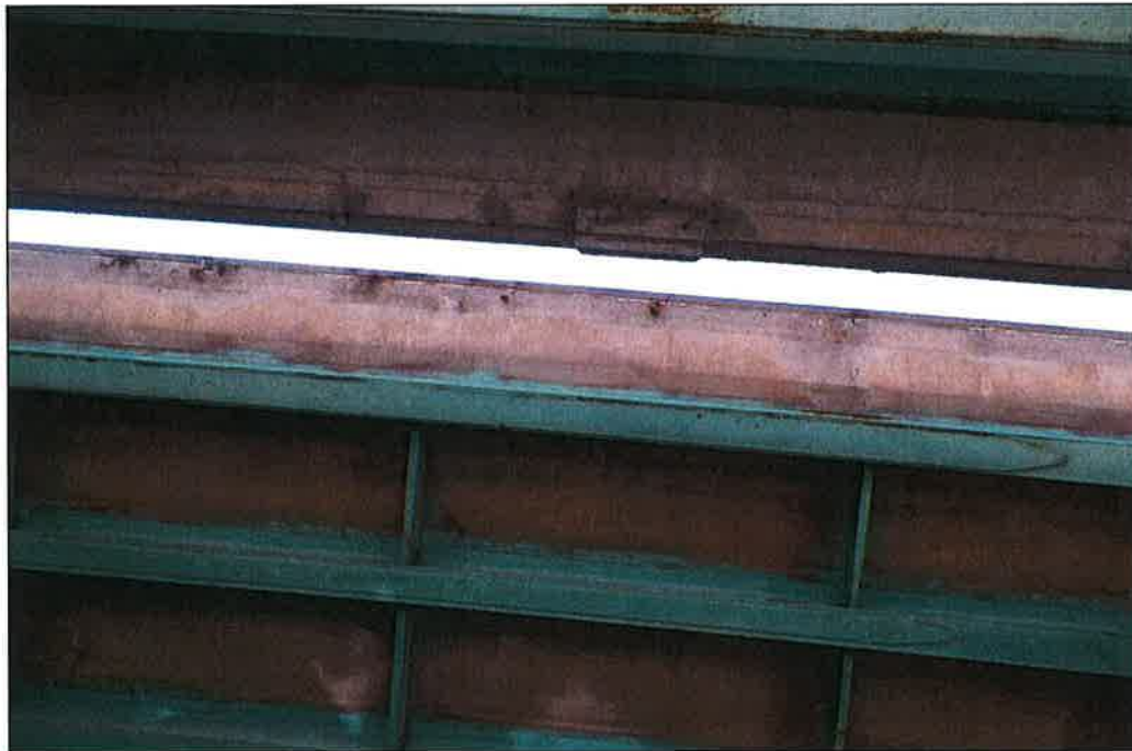
Photo P32 – Typical Condition of Fascia (Bent 120-121)
